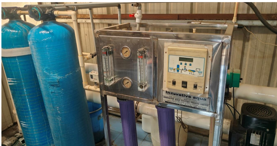
Figure 14: Revived and Functional RO Plant at Farhatabad
